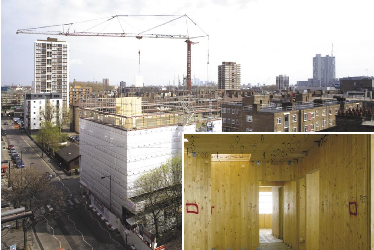
Opposite page and these photos: The Stradhaus is the UK's first timber panel tower. The nine-storey build is one of the first major UK housing projects to apply the middle European massive wood panelling system to an entire load-bearing structure.
